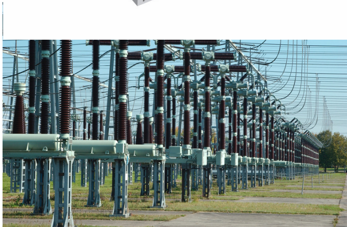
Power Utility Automation
