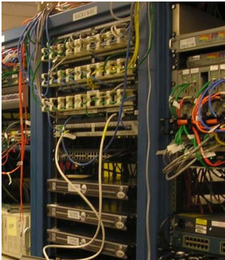
Rack view (front)
