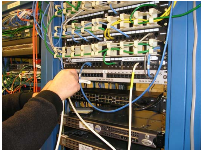
Rack view (front) close-up
