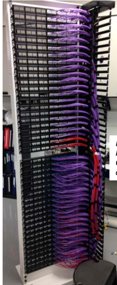
Patch Cord - Rack Under Test
