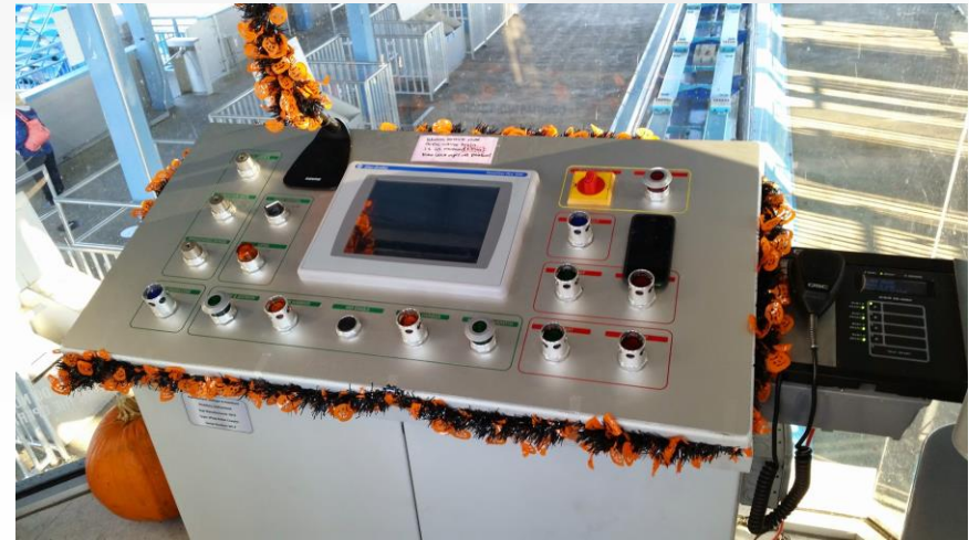
Amusement Park Operator Control Room
