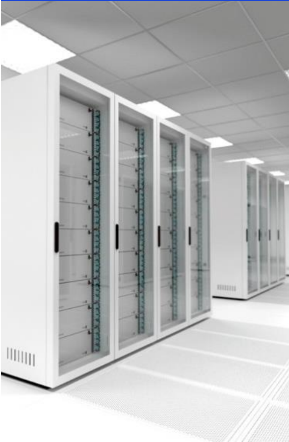
Inside the Data Center
